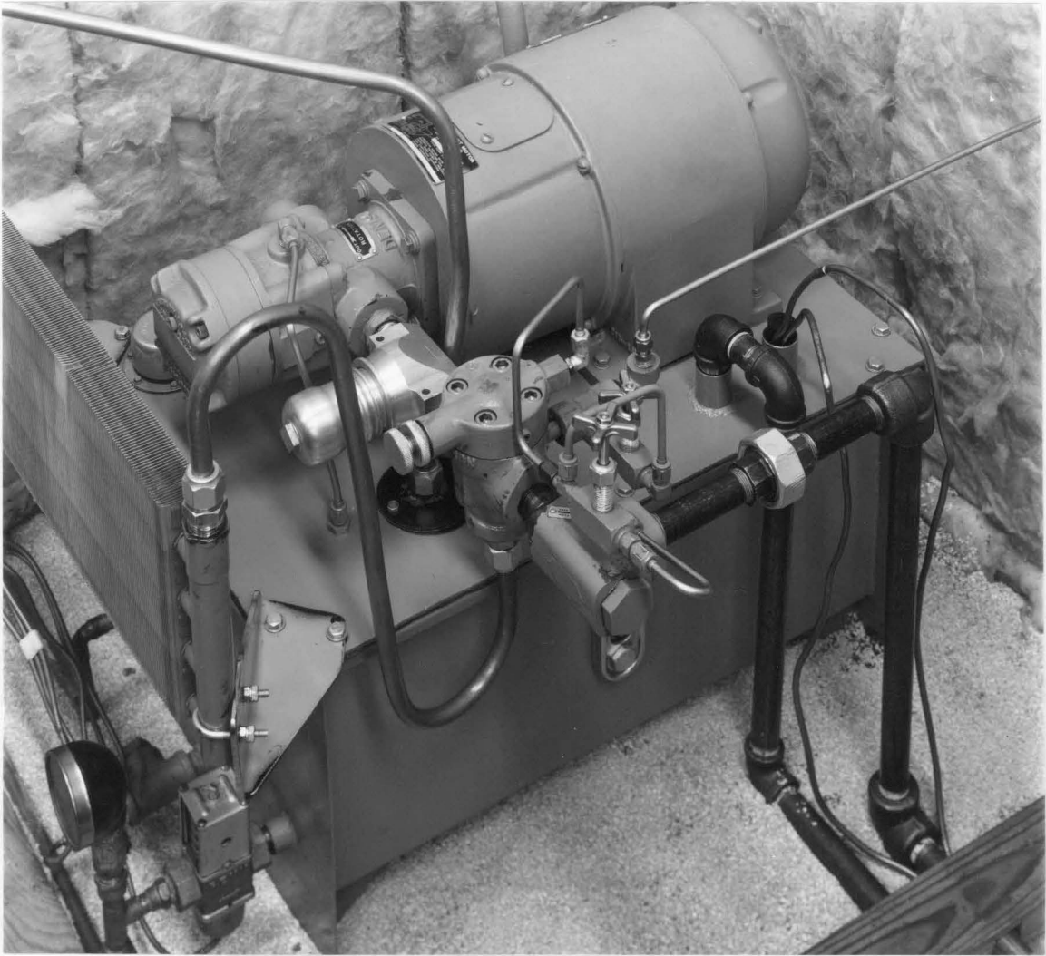
Fig. 4.7 View of the hydraulic supply unit.
