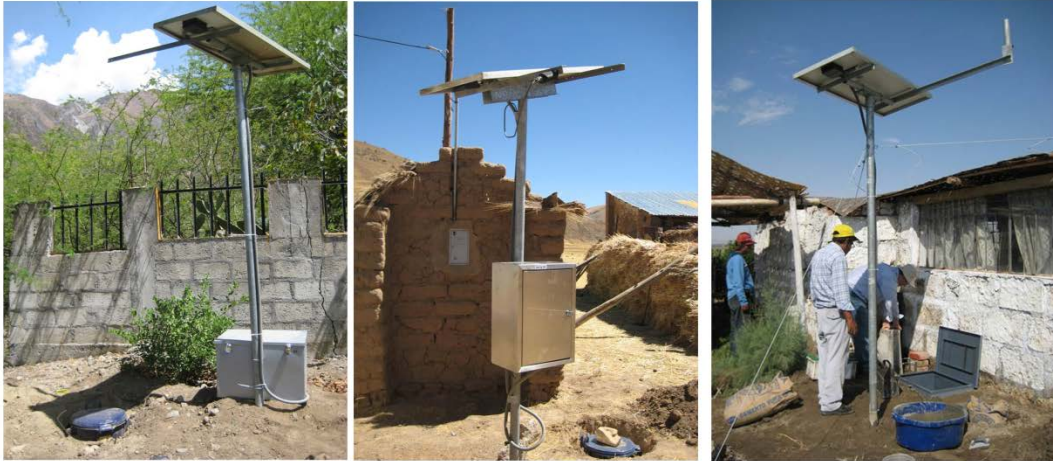
Figure 4.1: Photos from the installation of the seismic arrays. The sensor is placed in the round holes where a blue trashcan is visible. It is seated in a cement base and insulated. Power in these cases is supplied by solar panel, and the box containing equipment is either attached to the base of the mast (left), attached halfway up the mast (center), or buried in the ground (right).
