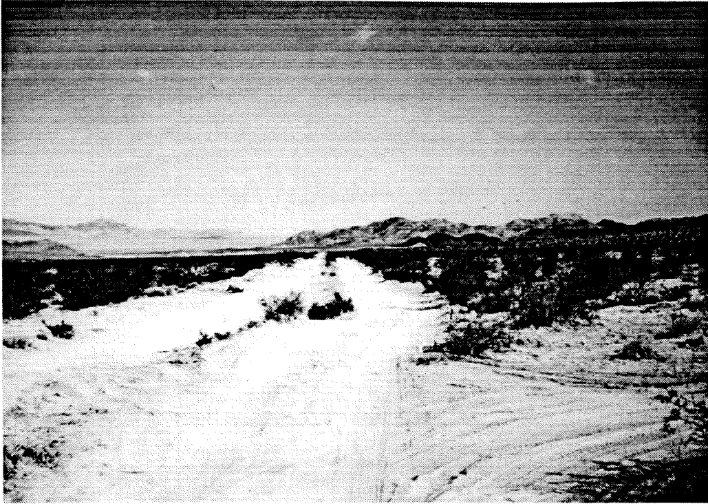
Figure 2.8 A Several Meter Horizontal Dislocation on a Road.
