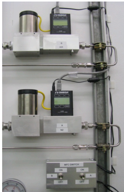
Figure 3.2: The mass flow controllers connected to the piping system
