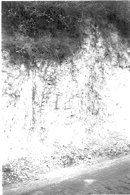
Fig. 15 Two zones of fault gouge along Whittier fault trace. On maintenance road 400' west of section CHI
