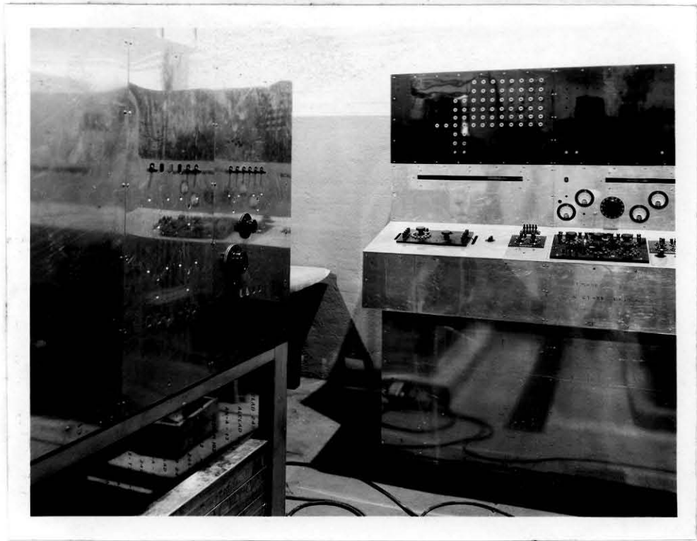
a) Electrical Panel of Volumetric Apparatus (Shown in Process of Construction) showing Location of Temperature Bench
