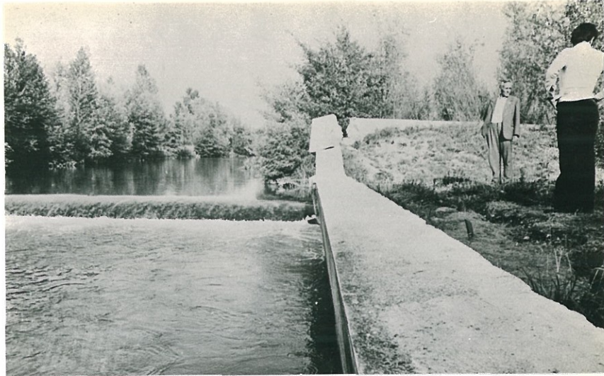
FIGURE 1.26 - WEIR ON THE LEDRA RIVER:DAMAGED RETAINING WALL - FROM (10)
