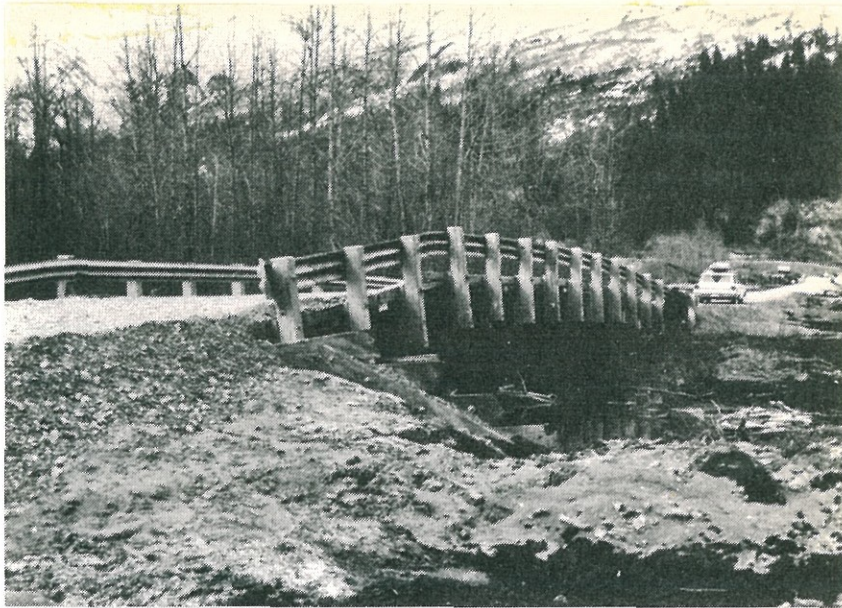
FIGURE 1.19 - SUPERSTRUCTURE BUCKLING OF SNOW RIVER BRIDGE 604 - FROM (45)
