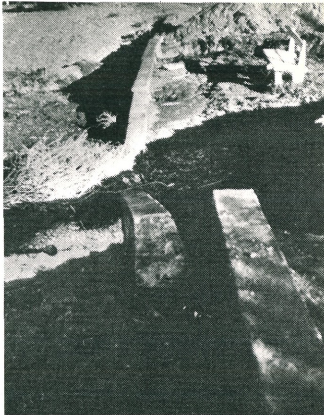
FIGURE 1.16 - FRUTILLAR, RETAINING WALL FAILURE - FROM (55)
