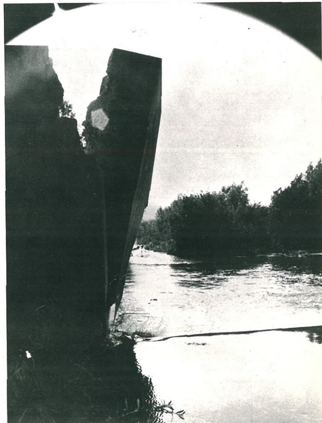
FIGURE 1.27 - WEIR ON THE LEDRA RIVER:DAMAGED RETAINING WALL - FROM (10)
