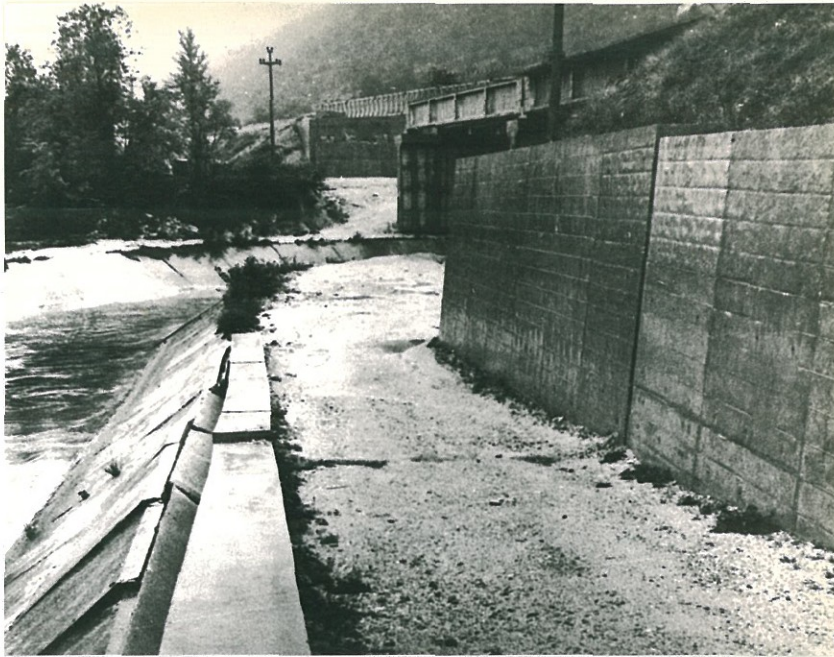
FIGURE 1.29 - DAMAGE TO EMBANKMENT RETAINING WALL AND CANAL, UDINE-CARNIA-TARVISIO HIGHWAY - FROM (I.C)
