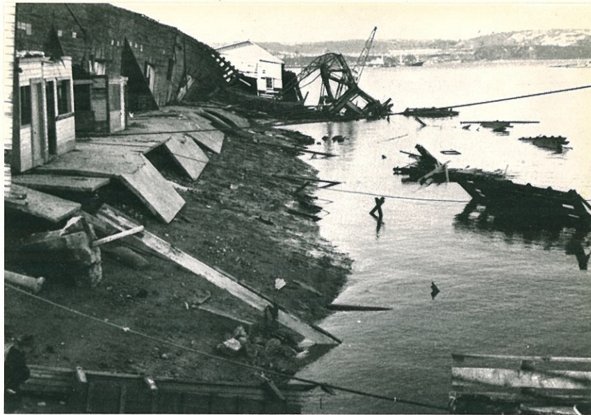
FIGURE 1.12 - FAILURE OF GRAVITY WALL AT PUERTO MONTT - FROM (11)
