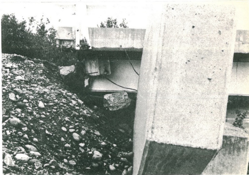
FIGURE 1.20 - SUPERSTRUCTURE DRIVEN THROUGH ABUTMENT BACKWALL, COPPER RIVER BRIDGE 345 - FROM (45)
