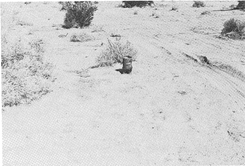
Figure 5: Photograph of the most deeply-buried vertical pipe on the flood irrigation system shown in figure 4.
