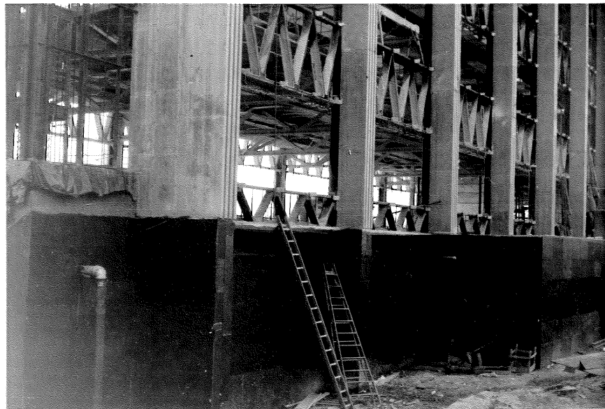
Fig. A-10 EXTERIOR VIEW, NORTH SIDE, SOIL UP TO 1st FLOOR LEVEL.
