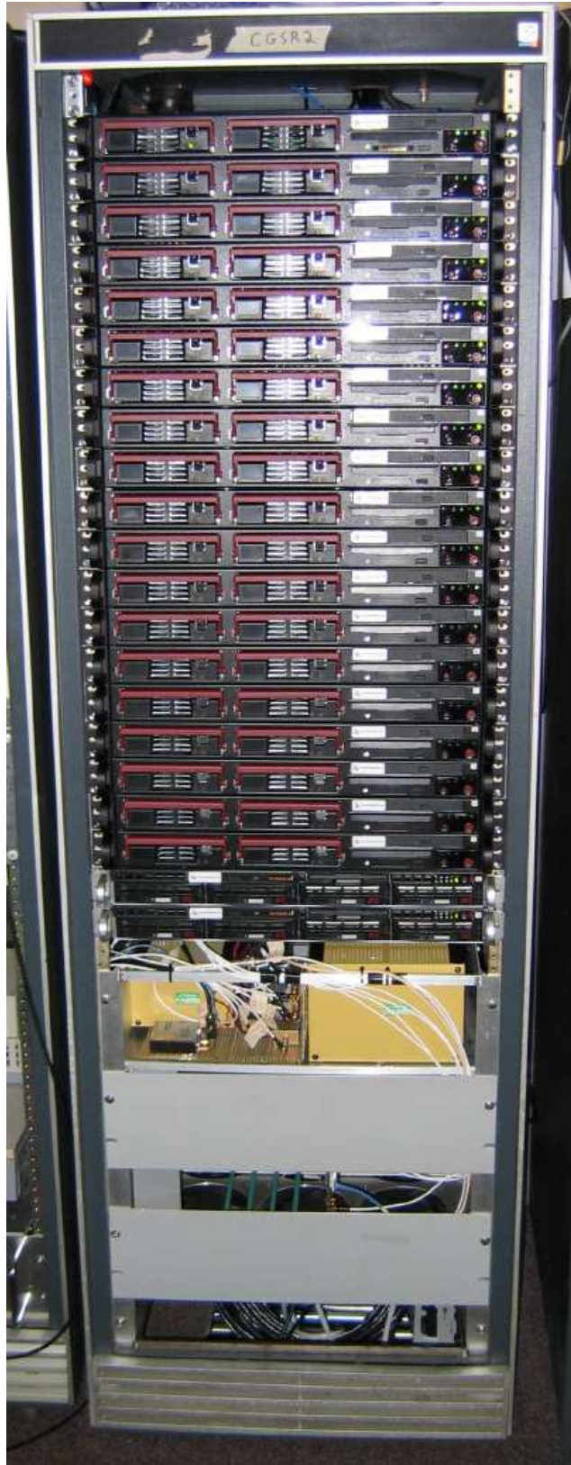
Figure B.4: Caltech – Green Bank – Swinburne Recorder II. The crate containing the FFD2, IF filters and amplifiers, 128 MHz sampler clock, and power supplies is at the bottom of the rack, below the dedicated computing cluster and Gb ethernet switch.
