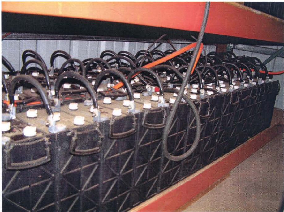
Figure 5-7 – Photograph of Backup Battery Bank
