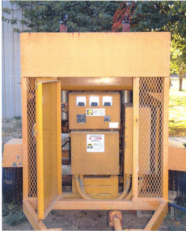
Figure 5-6 – Photograph of Generator
