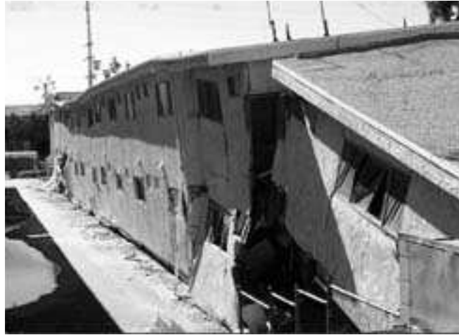
Figure 1.1: Northridge Apartments (collapse of 1st floor garage)
