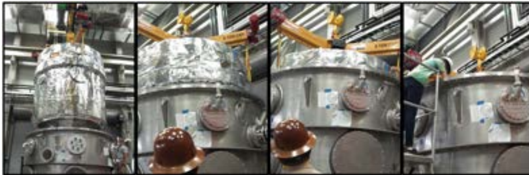
Figure 4.26: Nitrogen shield installation: a photo montage of the careful maneuver as the liquid nitrogen shield is lowered into the outer vacuum chamber and secured with cold mass support rods.
