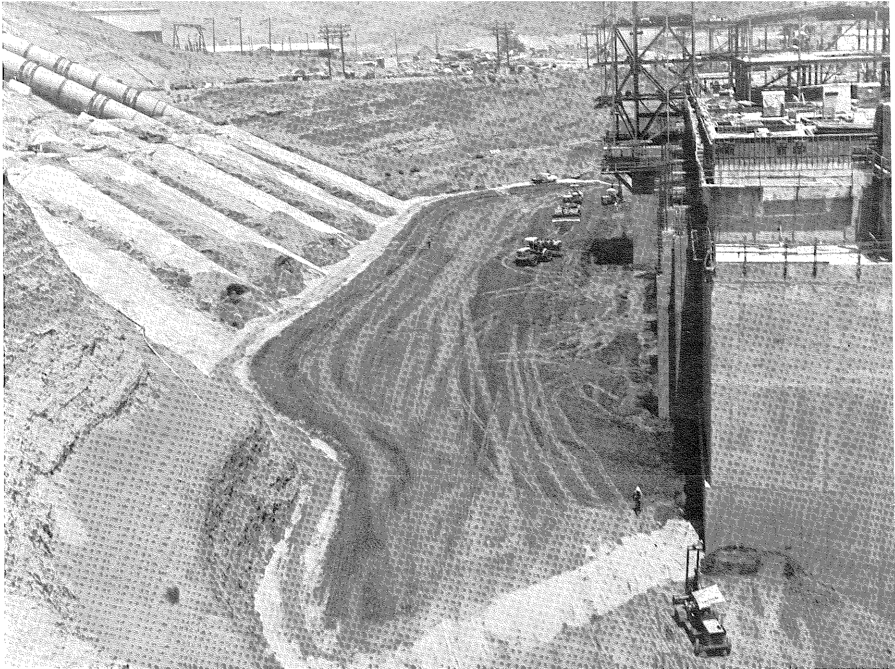
Figure 5.3 Castaic power-generating station under construction. Soil backfilling being placed against wall of structure.
