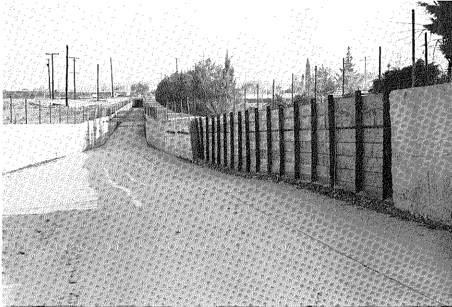
Figure 1.5 Lopez Canyon Channel. Temporary supports on failed section of wall.
