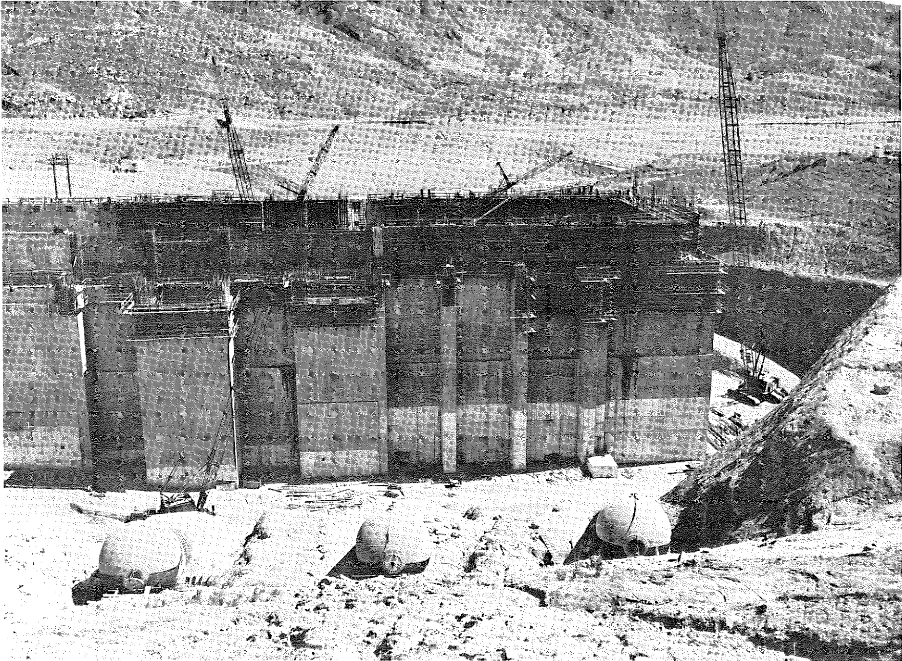
Figure 5.2 Castaic power-generating station under construction. Soil backfilling was placed between the wall in view and the penstock slope in the foreground.
