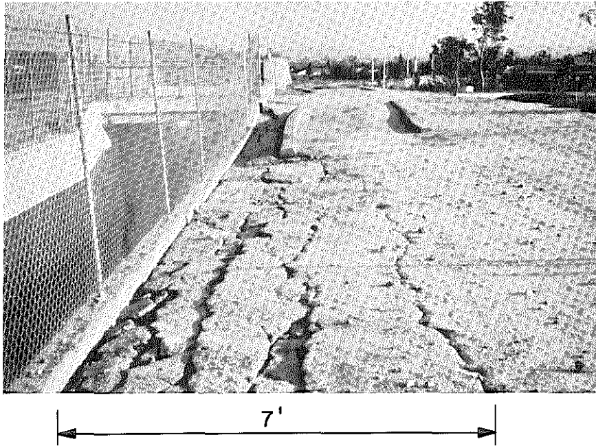
Figure 1.4 Wilson Canyon Channel. Cracking in soil as a result of wall displacements. Fine cracking was detected a distance of 15 ft behind wall.
