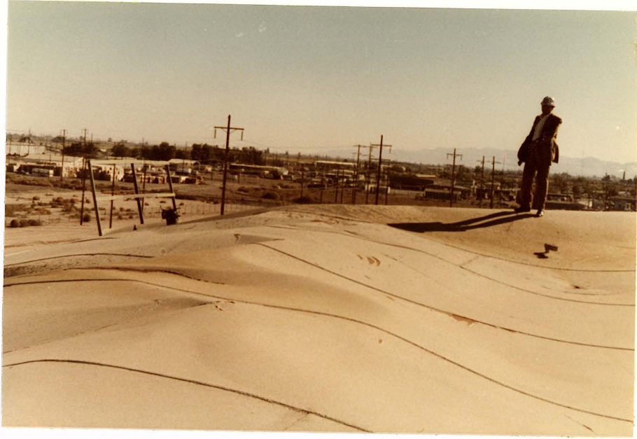
Fig. 1.4 DAMAGE ON ROOF OF TANK
