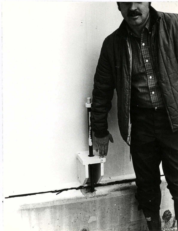
Fig. 1.5 UPLIFTING OF ANCHOR BOLT (COURTESY OF PAUL C. JENNINGS)
