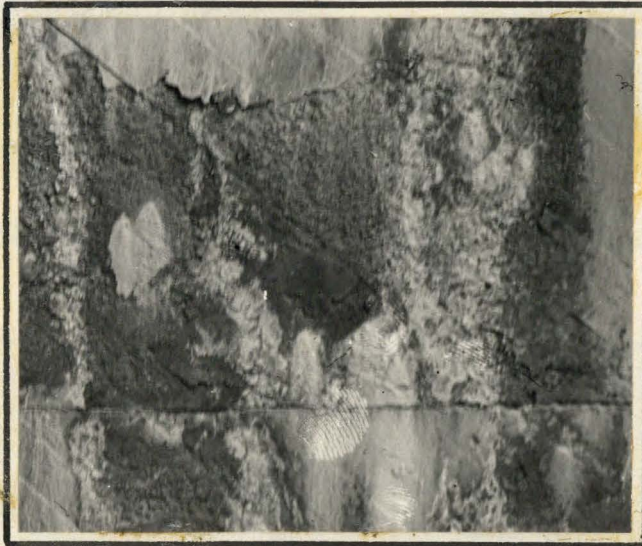
B. Exudations on concrete buttress No. 27 of Florence Lake Dam
