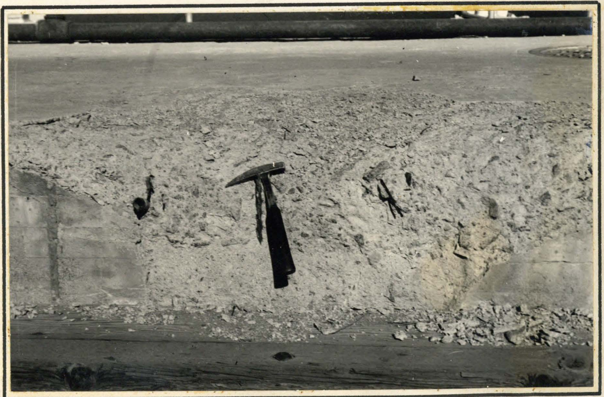
B. Deteriorated concrete of Huntington Lake Dam No. 1 "1917" aggregate was used. Typical of 1939 concrete failures also.
