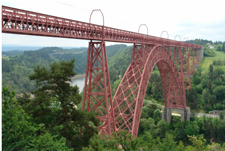
Figure 3.2: The Garabit Viaduct is another example of a structure with several levels of hierarchy. Image courtesy of Graeme Churchard taken from ( Garabit Viaduct 2009)
