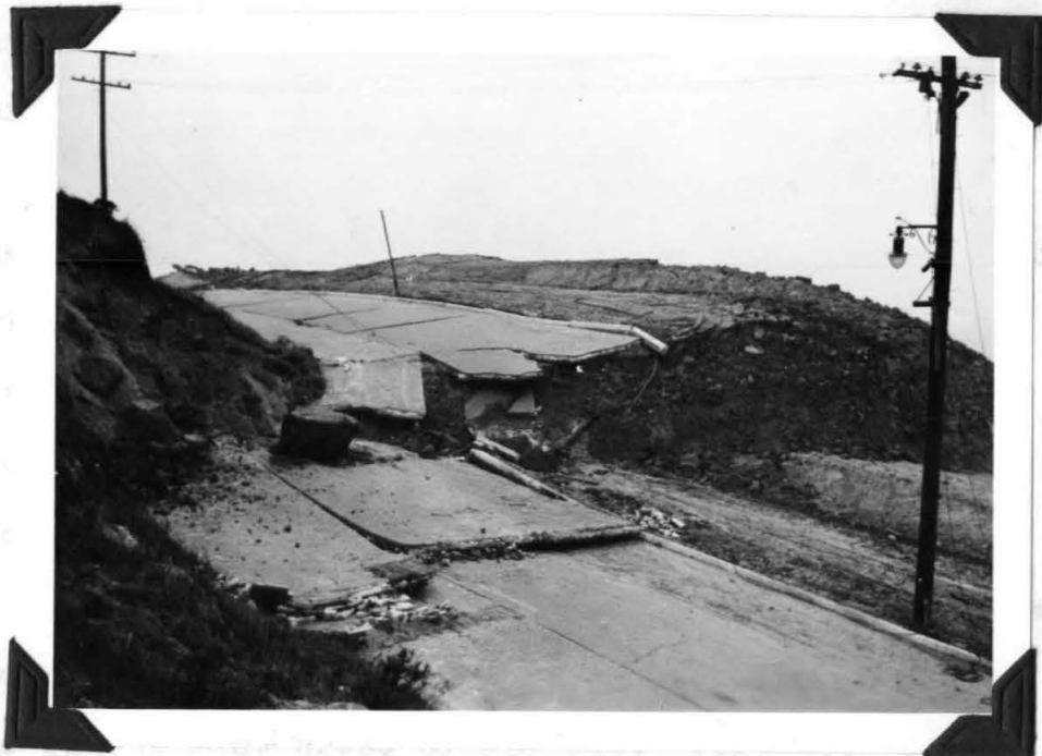
Fig. 13. Offset in pavement of Parker Avenue along northern edge of landslide.
